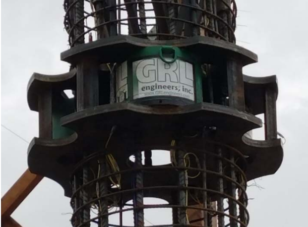
Fig. 2. Jack assembly, showing upper and lower bearing plates, and three 2,200-kip GRL-Cells
