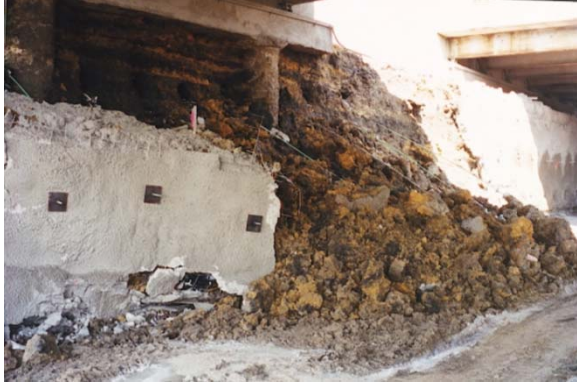
Figure 4: Failed Soil Wall System – It is evident the nails had insufficient grout coverage
