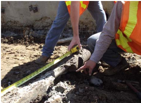
Figure 5: Insufficient Grout Coverage
