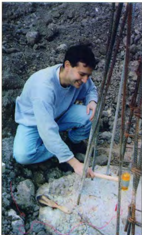
A technician strikes the cast-in-place concrete pile with a light hammer (above). The data from the resulting incident and reflected force wave is recorded in the Pile Integrity Tester recorder (below).
