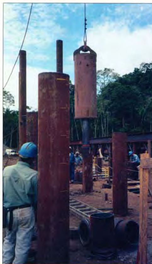
A large hammer strikes a driven pile while conducting dynamic pile monitoring.
