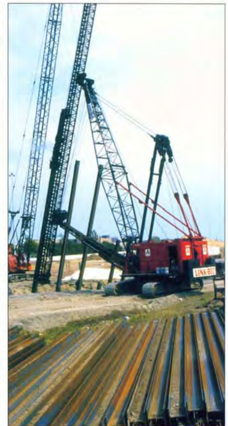
When continuous hammering produces insignificant movement at the pile toe, the load carrying capacity has been achieved.
