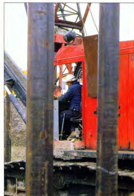
A close-up of steel pipe pile and the cab of crane for pile driving equipment.
