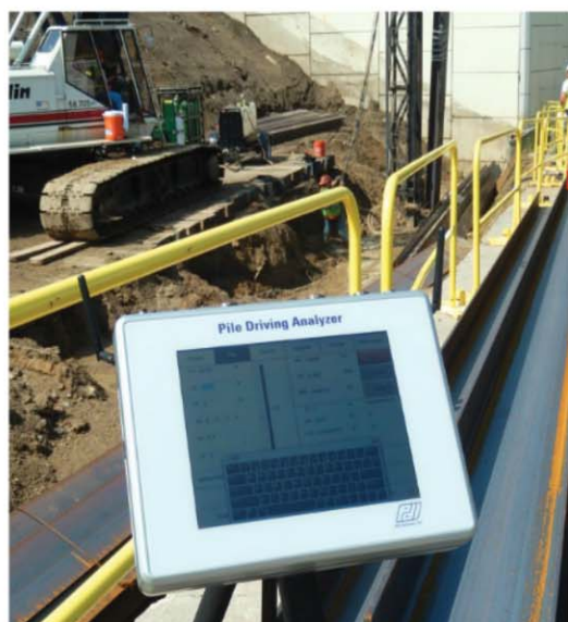
PDA-8G in use to monitor installation of driven piles on the Eastbound span of the George V. Voinovich Bridge (commonly known as Innerbelt Bridge), which spans the Cuyahoga River on Interstate 90 in Cleveland, Ohio
