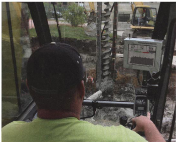
The main module of Pile Dynamic's installation recorder in the operator's cabin.
