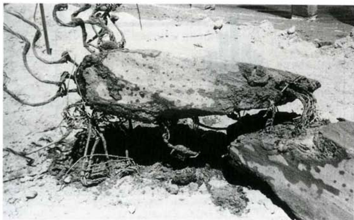
Figure 7: Damaged Prestressed Concrete Pile
