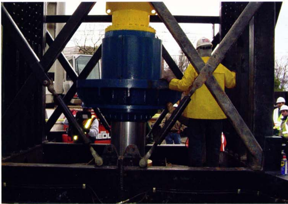
Figure 5: Statnamic Piton (with load cell and displacement sensor) mounted on top of shaft, Stratford, CT
