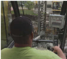
The new PIR displays the incremental grout volume and other variables that are essential for QA/QC on a much more visible screen.
