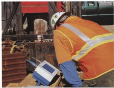
Figure 4 - APPLE (red ram) and Pile Driving Analyzer (blue and white instrument) used in dynamic load testing.
