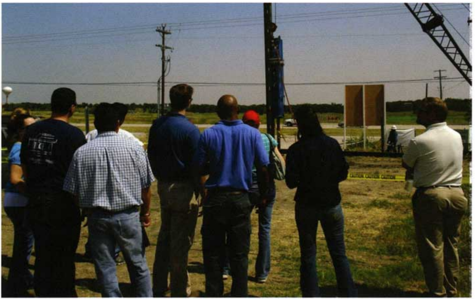
The Pile Master 36-3000 driving a 6-5/8 inch, 25 ft long pipe pile in Manor, TX
