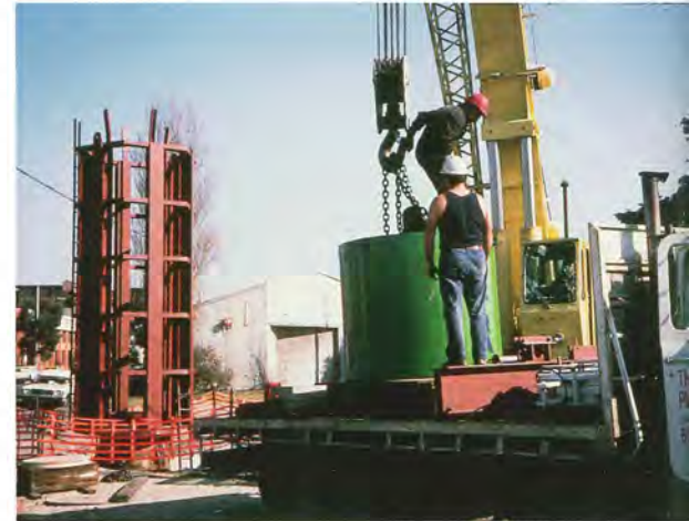
Drop weight used to test cast-in-place shafts at the West Gate Freeway project in Melbourne, Australia
