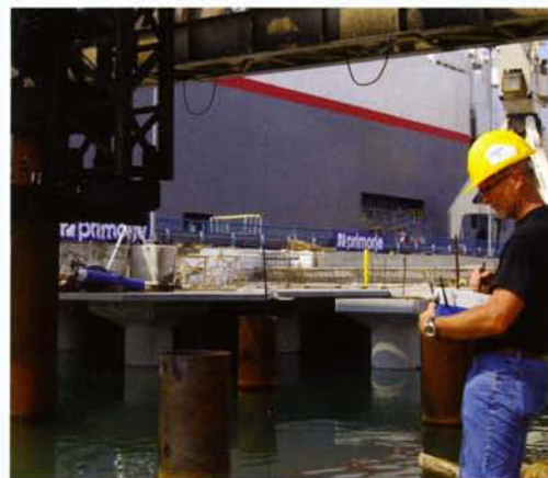
Load tests are being carried out on the pile foundations installed for the construction of a new pier at the Port of Koper in Slovenia using a Pile Dynamics' PAX Wireless Pile Driving Analyzer (PDA) model.
