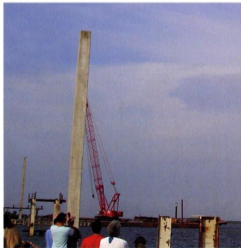
GRL Engineers is carrying out dynamic load testing on the piles for the replacement Max Brewer Bridge crossing the Indian River in Florida, US.
